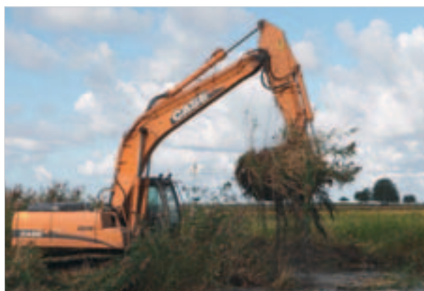
Photo 6.1.8. Removal of reed and its thick rhizome layer with a digger from the northern shore of the large lagoon of Vöiste in 2009.
