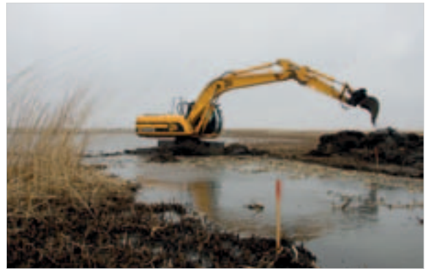
Photo 6.1.5. Restoration of a sea connection channel of a coastal lagoon with a digger
